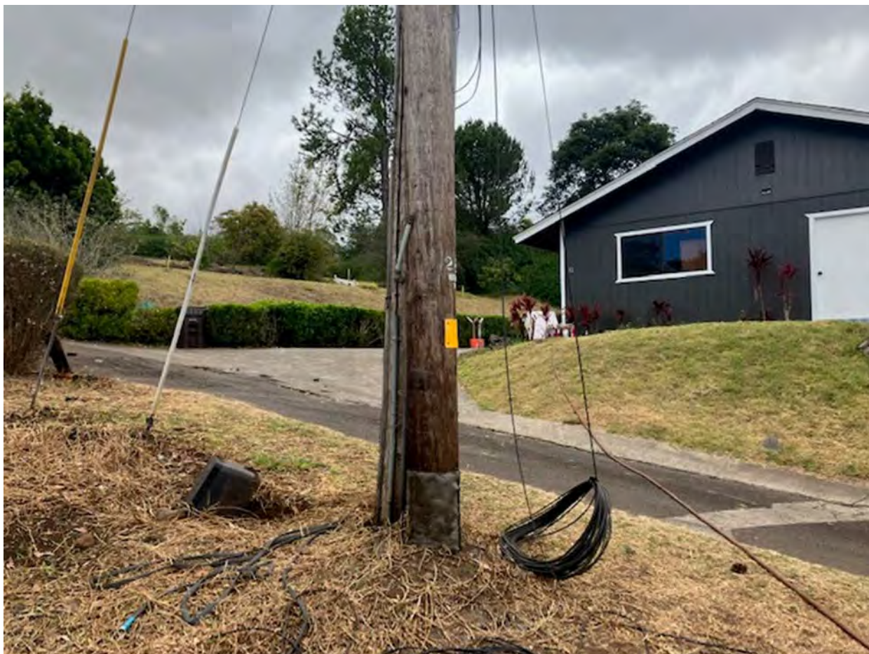
Figure 3: Pole 28, the suspected ignition source of the Kula Fire.
