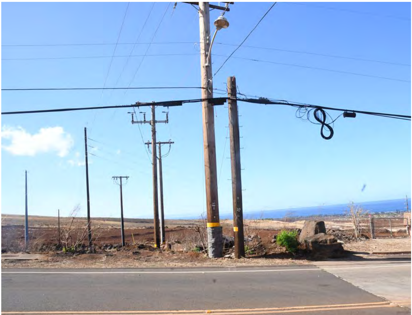
Figure 5: Pole 25, the suspected ignition point of the Lahaina Fire.
